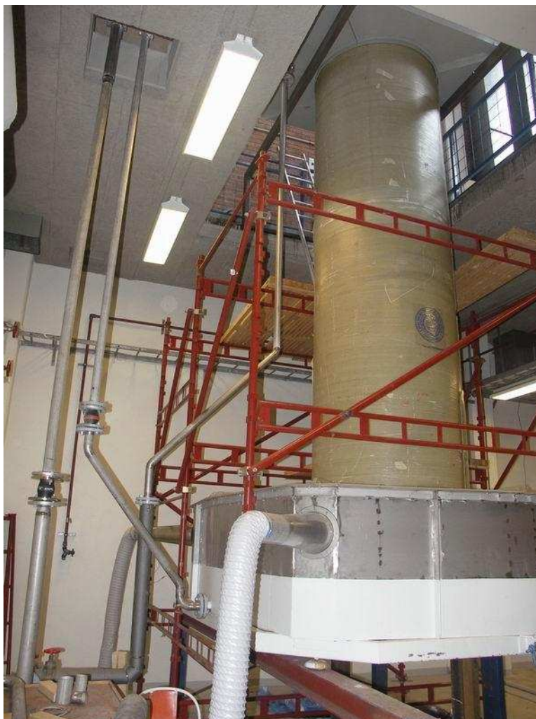
Figure 2.6: Natural convection rig; hot water piping and air circulation housings.
